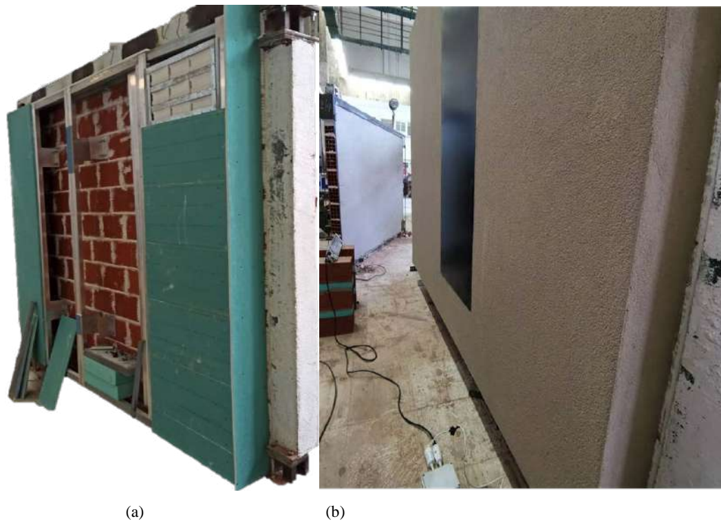
Figure 2. Presentation of under evaluation ventilated facade, (a) construction phase and (b) final configuration, PV mounted, radiation lamp and automation installed.
