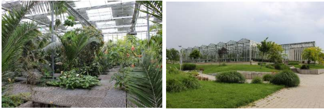
Figure 5. Figure 5. South Pest Wastewater treatment facility (Budapest, 2012, architecture authorship unknown to us): Plants grown in controlled environment assist in the process of aerobic/oxygenated fixed-film waste water treatment.) Photo: paper's first author
