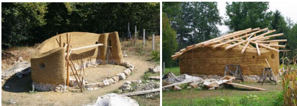
Figure 10. (Half)greenhouse, Banja Luka, Republic of Srpska, Bosnia and Herzegovina (arch. papers first author, 2011-2014) during construction of the heat-retaining northern wall and roof structure. Materials: earth, straw, wood, glass. Photo: paper's first author
